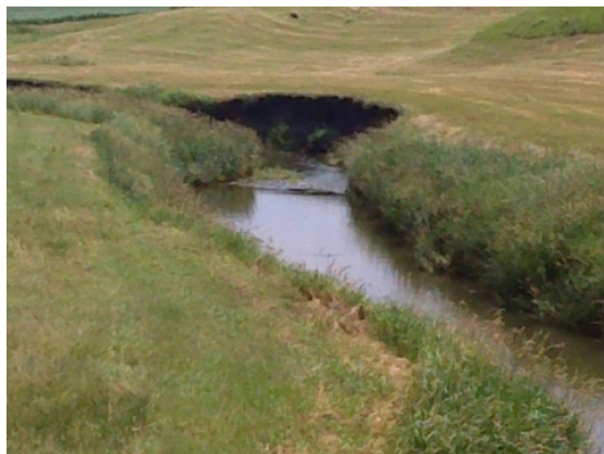
Figure 18: Eroded bank at 11MS040 along Upper Beaver Creek (10170203-521)
