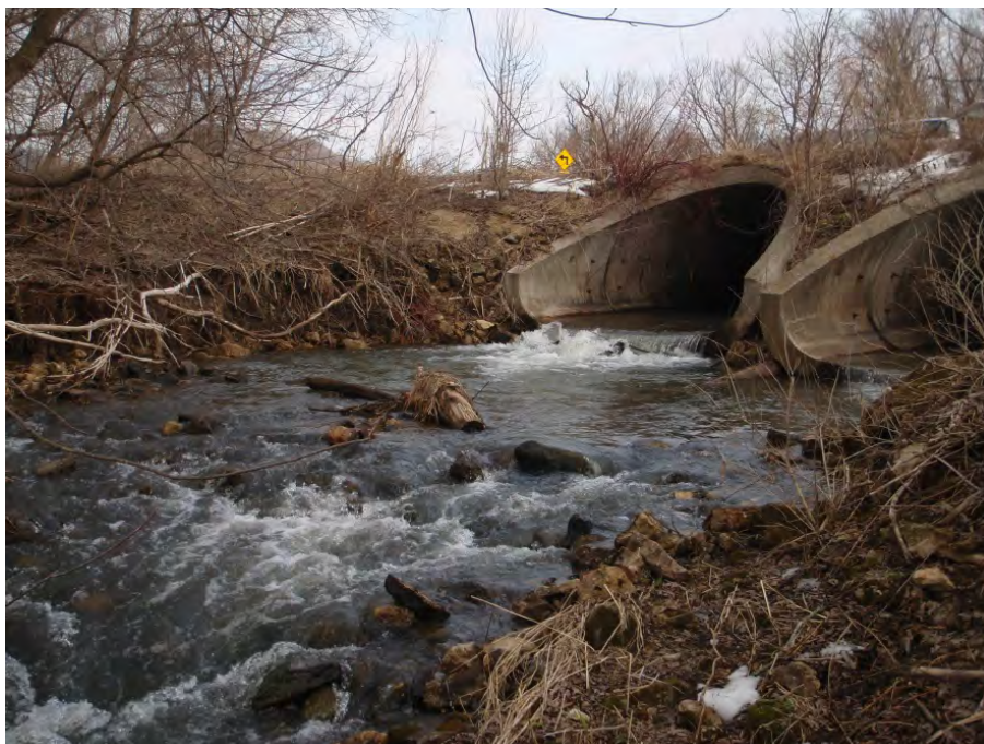
Figure 65. Perched culvert at CR17 and Station 08LM018. MPCA photograph March 18, 2011.
