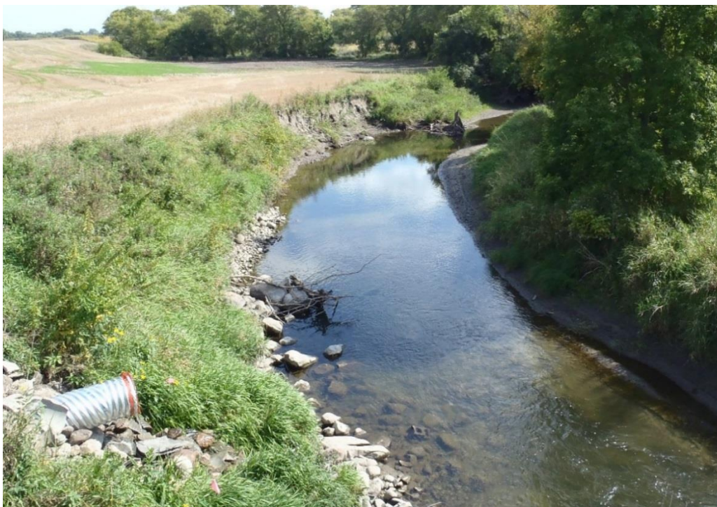
Figure 45. Bank erosion at station 15MN049 (9/18/14)
