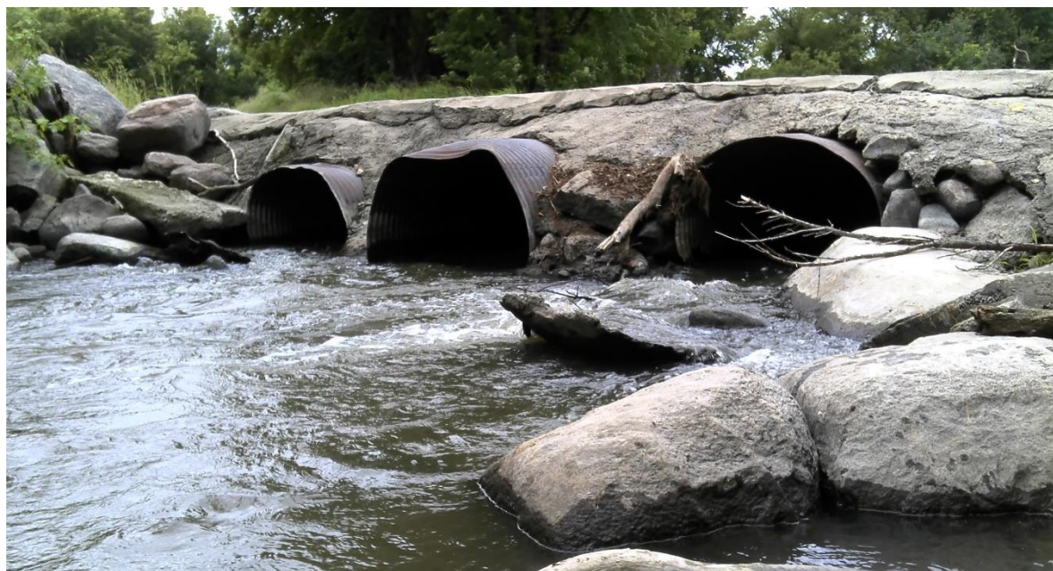
Figure 90. Undersized culvert on the West Branch Lac qui Parle River (photo credit DNR)
