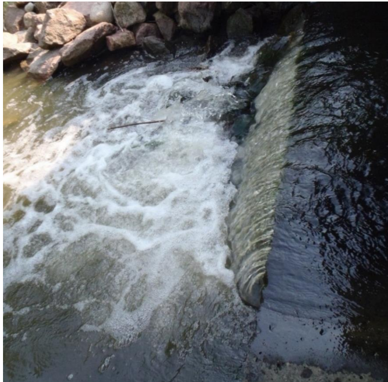
Figure 83. Perched culvert at site 09MN090
