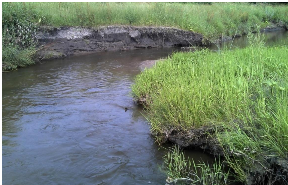
Figure 43. Bank erosion at station 15MN045 (7/8/15)
