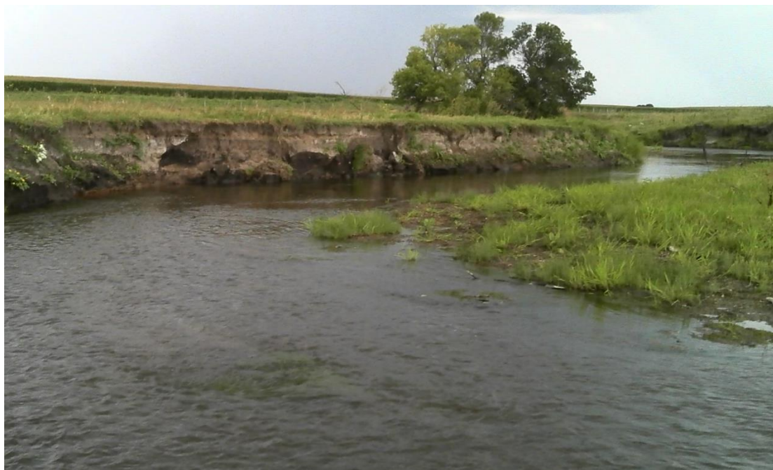
Figure 20. Erosion at site 15MN074 (8/13/15)
