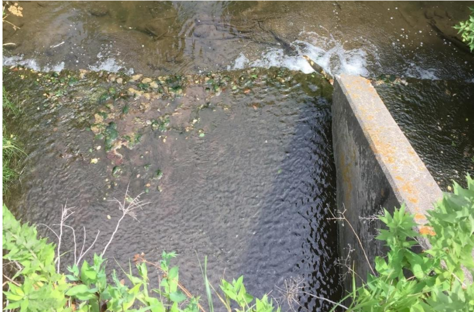
Figure 46. Perched culvert at station 09MN093
