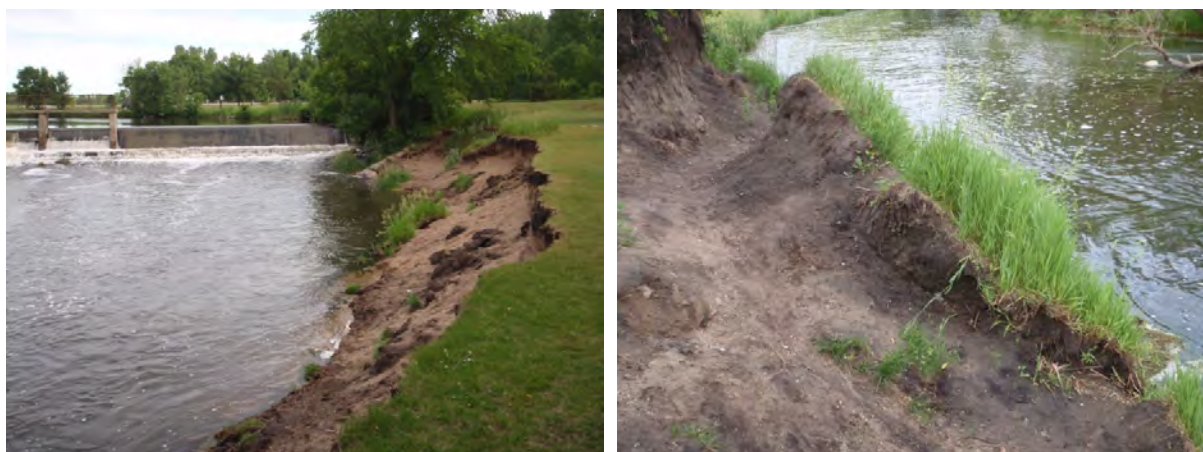
Figure 90. Photographs showing streambanks below Morris dam
