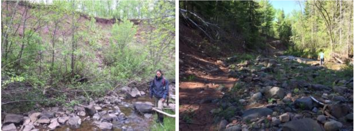
Figure 12. Category 5 Erosion Rates Observed in Reaches AM-3 and AM-2 (less than 0.1 ft/yr streambank erosion and variable hillslope erosion rates).
