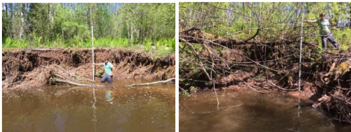
Figure 11. Category 4 Erosion Rates Observed in Reaches AM-9 and AM-10 (0.5 to 2.0 ft/yr).
