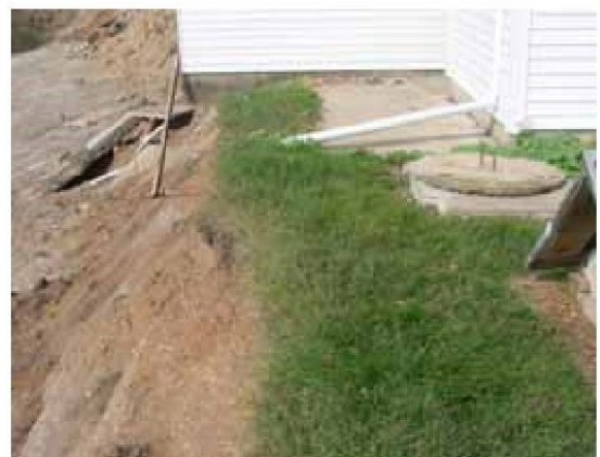
Washed away SSTs in eroded stream bank
