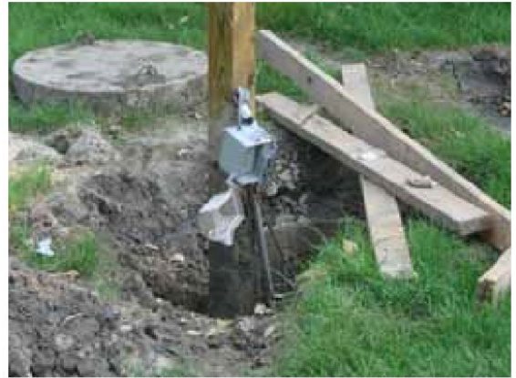
Flood damaged SSTS electrical box
