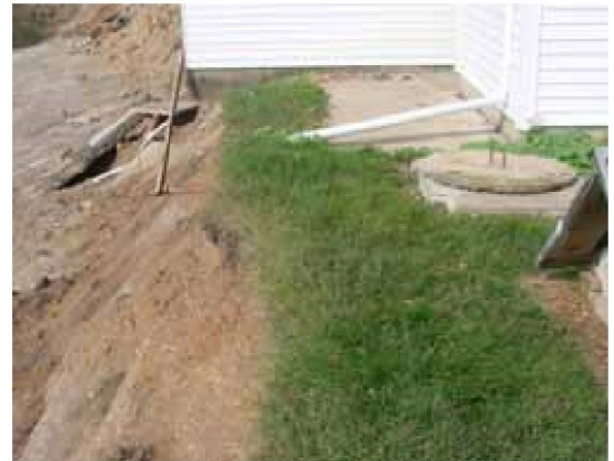
Washed away SSTS in eroded stream bank
